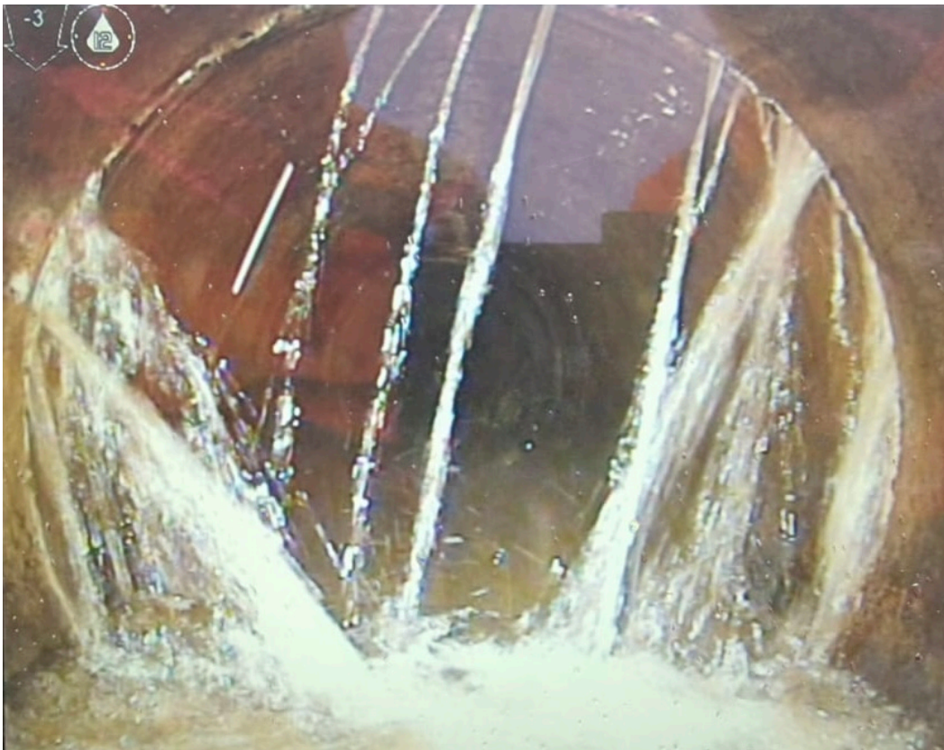
Monxton High Street - Groundwater entering the sewer via a pipe joint (July 2022)
